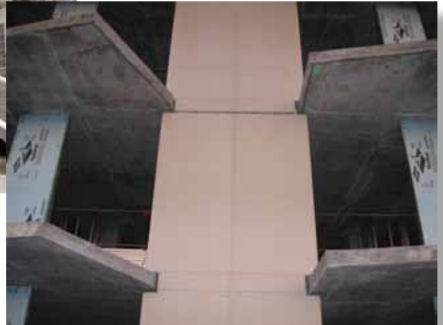
Architectural precast concrete wall panels at the new Armed Forces Retirement Home were designed to fit snugly around balconies and other projections. The design is the first along the Mississippi coast designed to withstand winds of more than 200 mph in a Category 5 hurricane.
